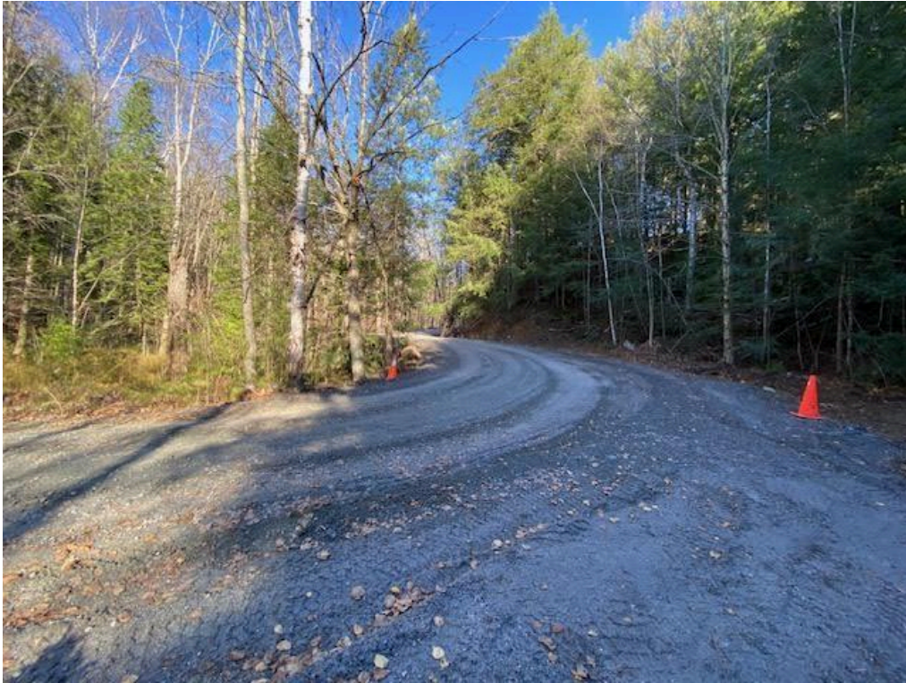
Photograph 3: Example of road widening beside tributary; culvert under road out of photo on left
